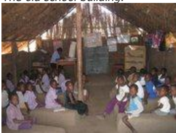
Taken inside in 2009 - the building has deteriorated beyond repa
