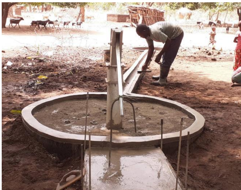
Putting the finishing touches to the Chilepa borehole, run off, surround and garden pond.
