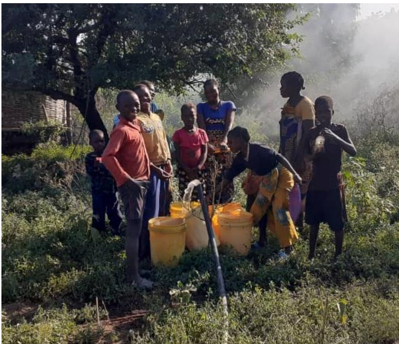
Great excitement as the first clean water is pumped during the 'pump test'
