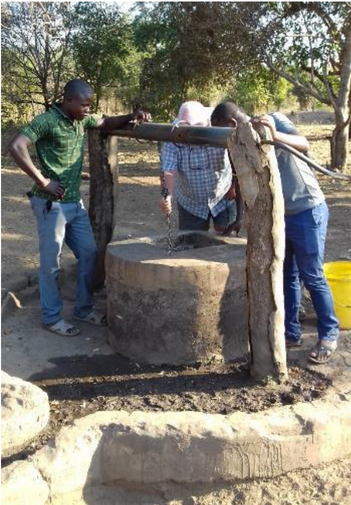
The dysfunctional well at Chimanga
