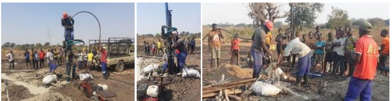
Drilling at Kambwi – with a lot of help and interest from the community.
