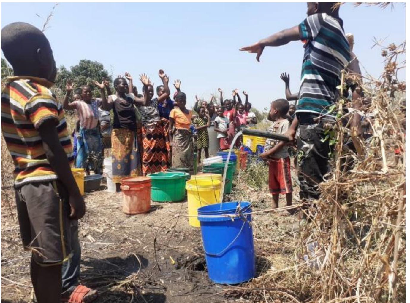
Absolute delight and excitement when the first water is pumped from the new borehole at Nsambwa!
