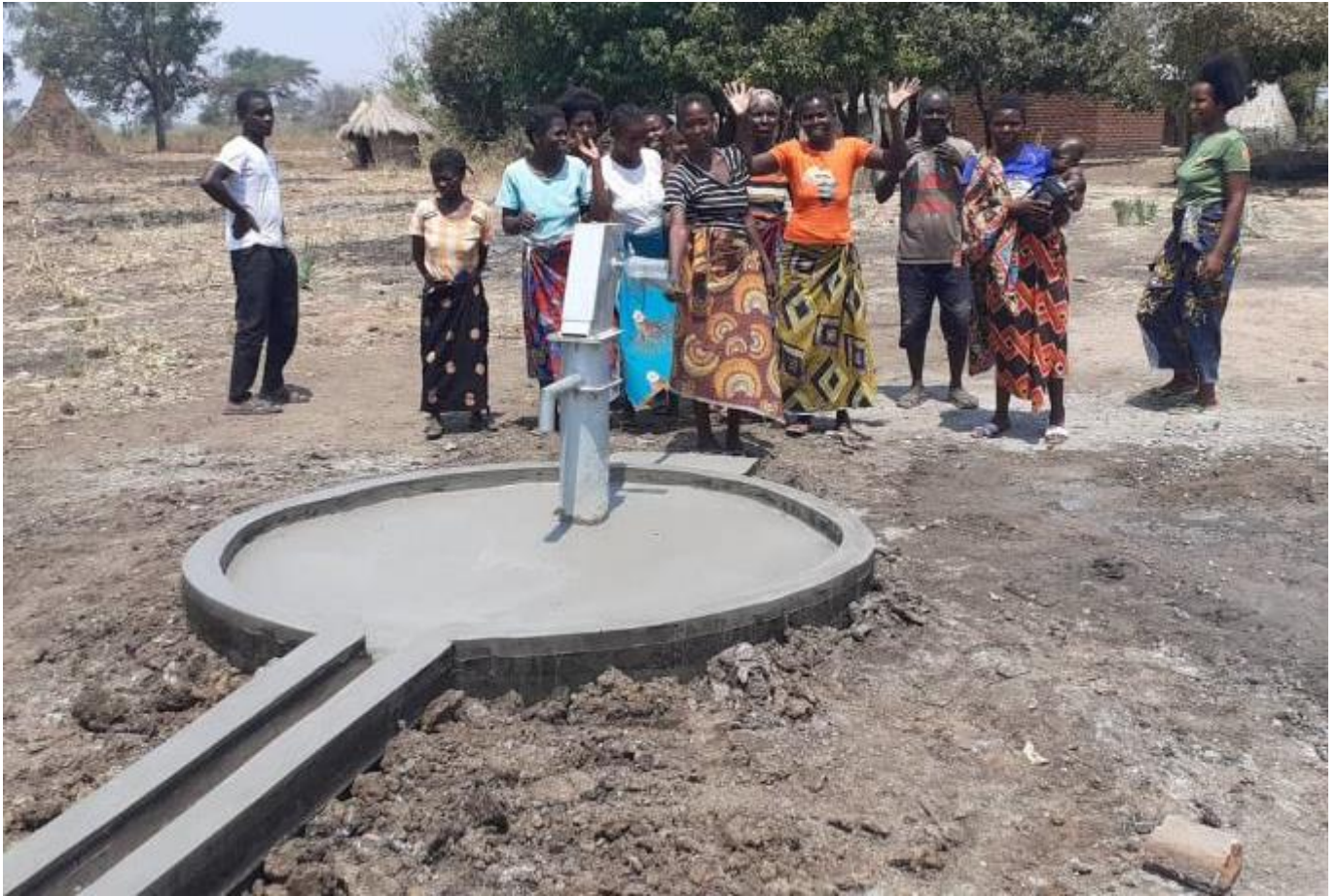
Finally Nsambwa has their new complete borehole – just waiting for the concrete to dry – then it can be used.
