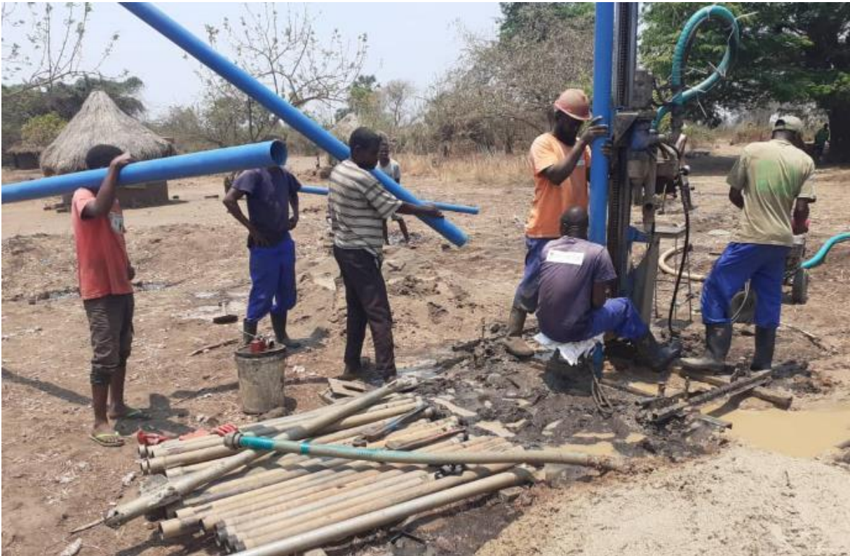
Some very welcome volunteers help the team install the casing at M'Longoti.
